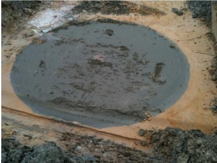
Figure 6 Shows a soil mixed column through sandy ground, note how the binder is defined to a specific area and does not spread to the surrounding ground. Photo courtesy of Deep Soil Mixing
