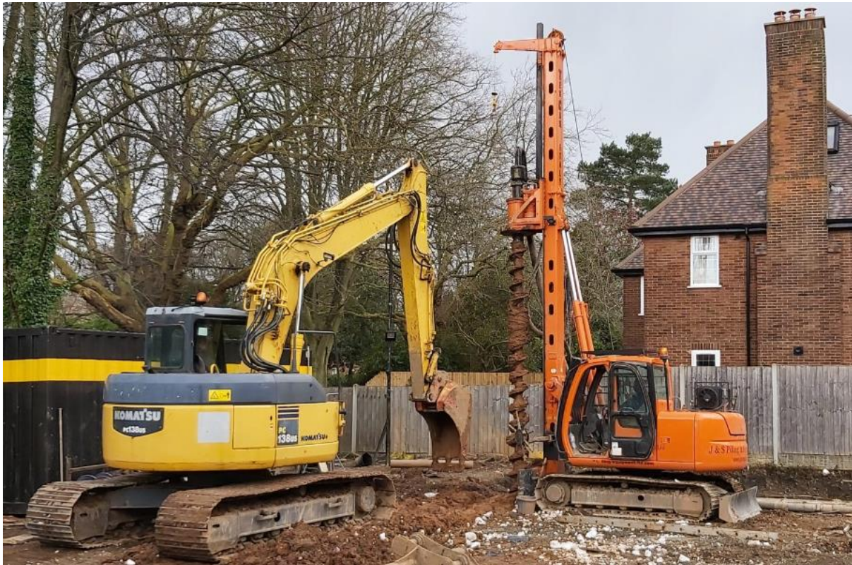
Figure 9 10t excavator with piling rig attachment for installing continuous flight augured piles.
