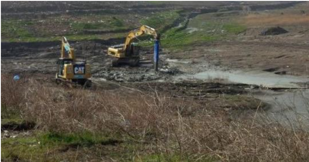
Figure 3 An example of soil mixing taking place. Photo courtesy of Deep Soil Mixing
