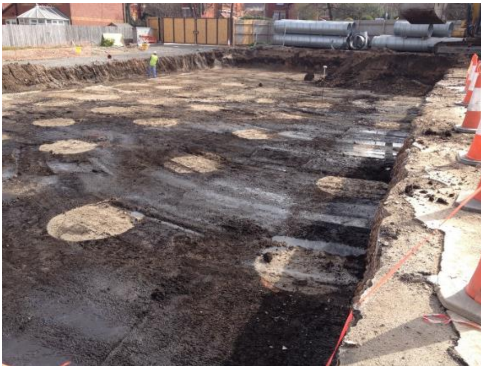
Figure 7 Soil mixed columns coloured in cream, with little to no mitigation of the added binder to the surrounding ground. Photo courtesy of xxxx
