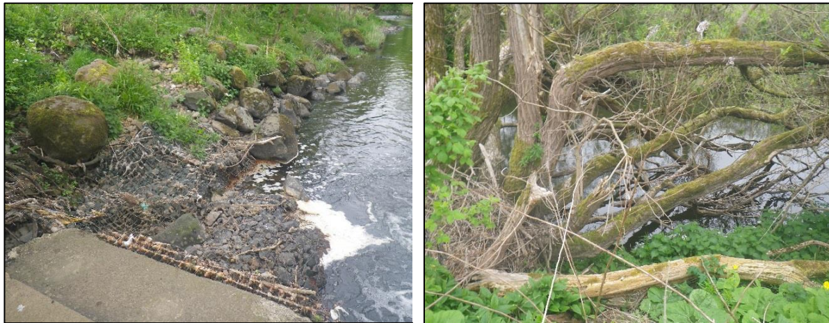
Plates 4.1 – 4.4: Lateral bars (top left), Actively eroding banks (top right). Failure of weir and bank (bottom left) and localised bank erosion and wood in channel (bottom right)
