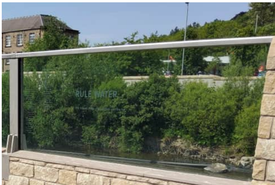
Figure 76: Example of etching on glass (note - this barrier is not a flood wall)
