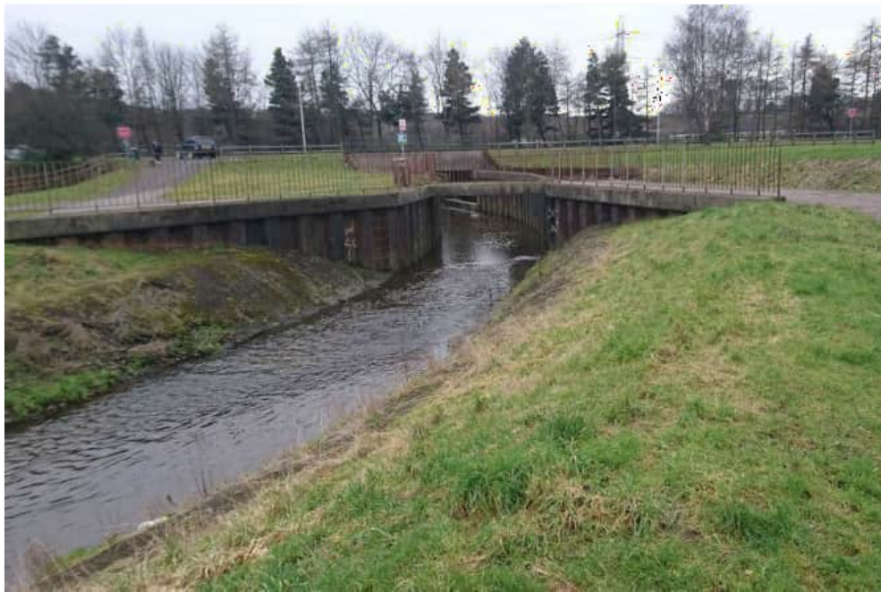
Figure 3-23: View looking south toward location of proposed flow control structure (GR: NS 92621 79866)
